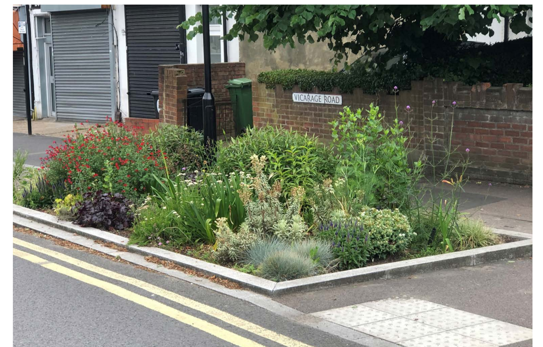
Typical porous asphalt and rain garden
