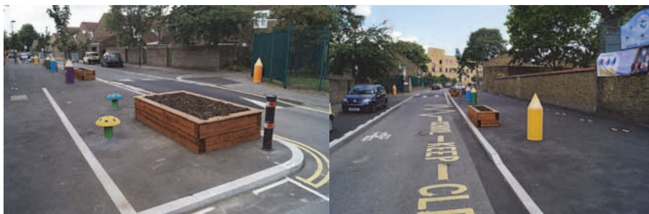
Narrowing of road outside a school in Lambeth to provide space for children and prevent parents parking in school keep clear area
