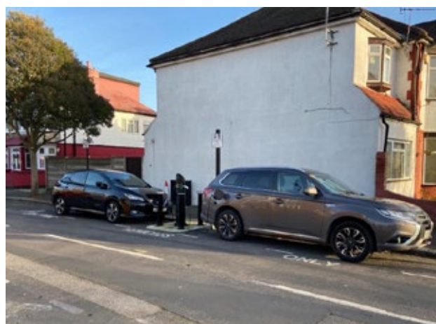
A freestanding electric vehicle charging point on Burchell Road, Leyton
