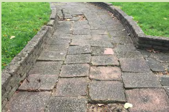
Paving in poor condition at Chingford Road open space.
